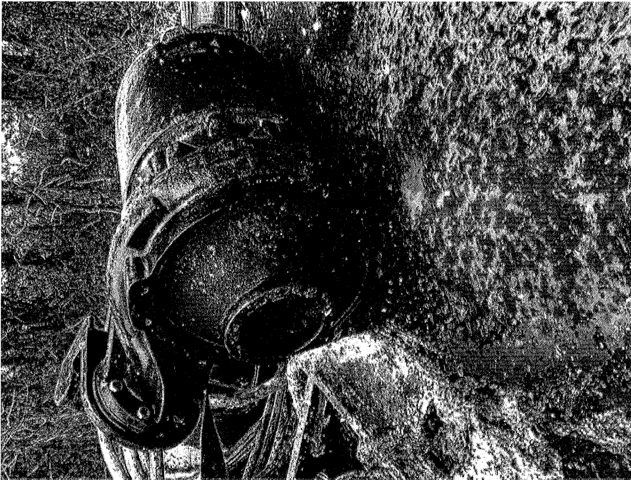
Pump with broken suction plate "volute"
