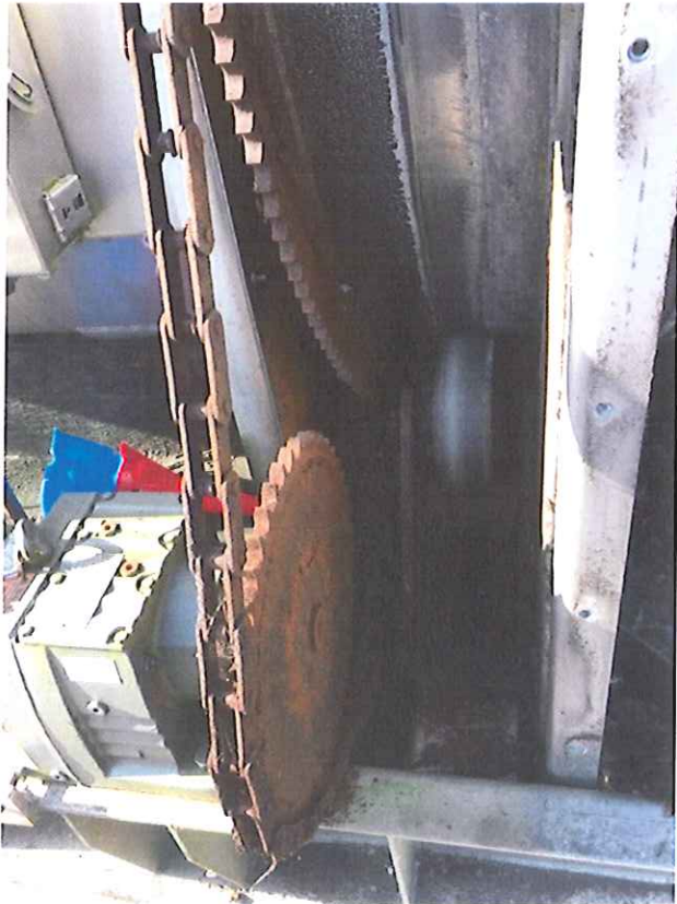
Corroded drive spur gear, drum gear teeth, and chain.
