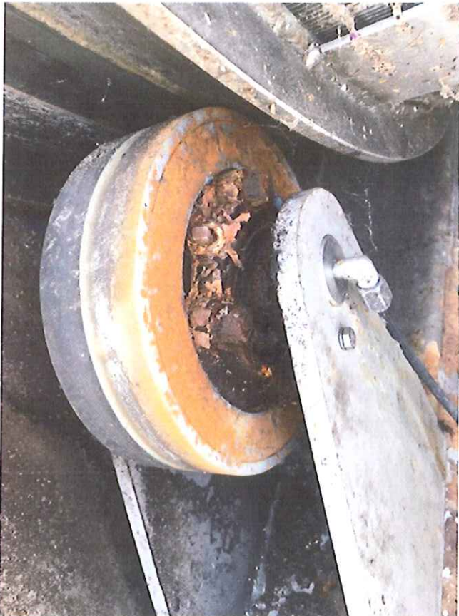
Corroded trunnion bearings.
