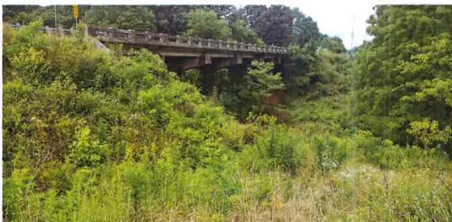
DATE TAKEN: 7/20/2021 VIEW WEST PROPOSED WESTERN FEE ACQUISITION AREA AND PROPOSED BRIDGE REPLACEMENT
